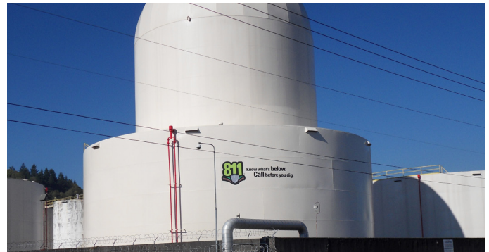
Energy product storage tanks, like these from Phillips 66 Pipeline LLC, are large canvases for the 811 logo.
